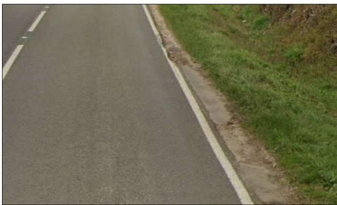
Figure 4 – B4525 typical verge over-run and damage to edge of carriageway. Evidence of previous edge of carriageway strengthening.
