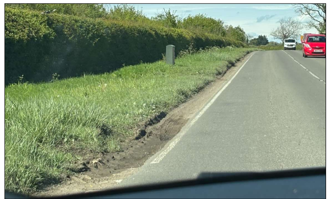
Figure 5 - B4525 typical verge over-run and damage to edge of carriageway with significant rutting in the verge.
