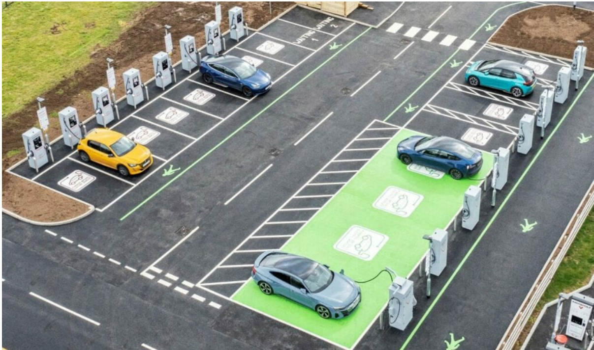
Figure 2: Example of a Charging Hub
