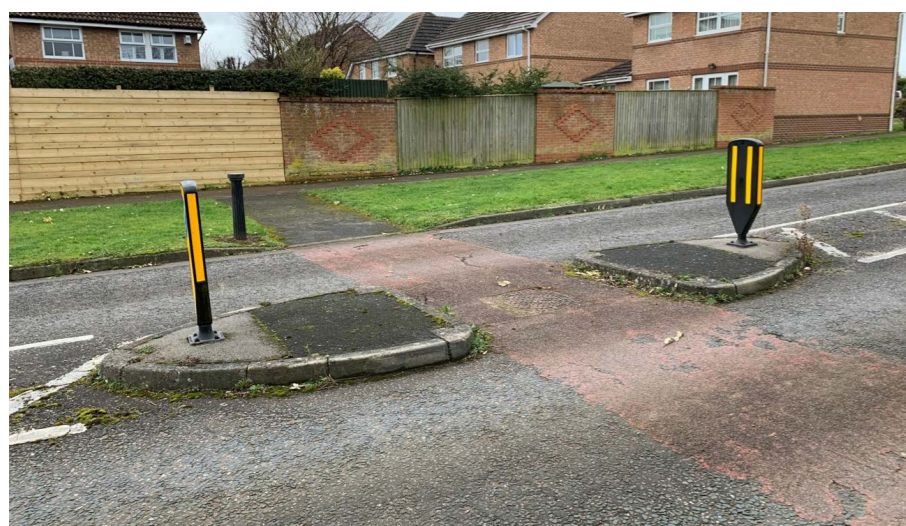
Lack of dropped kerbs
