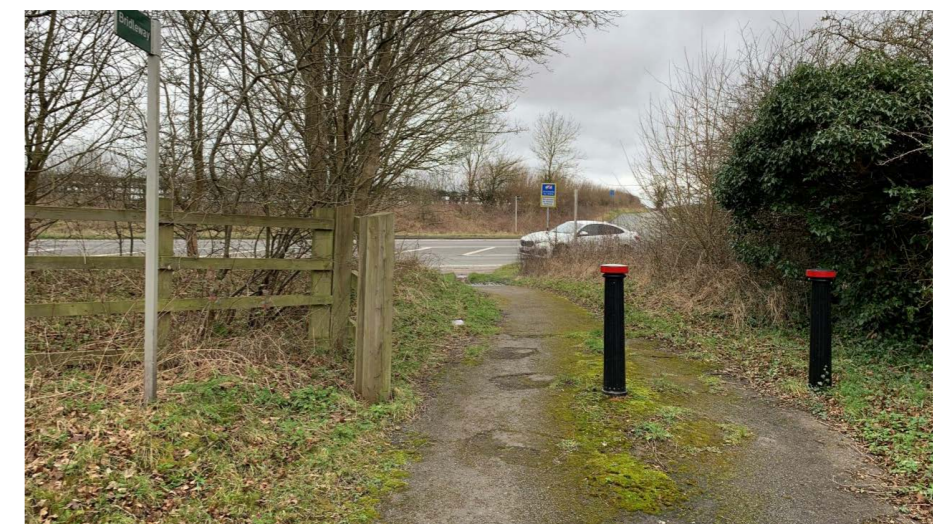
Existing modal filtered path from the A422 requires resurfacing
