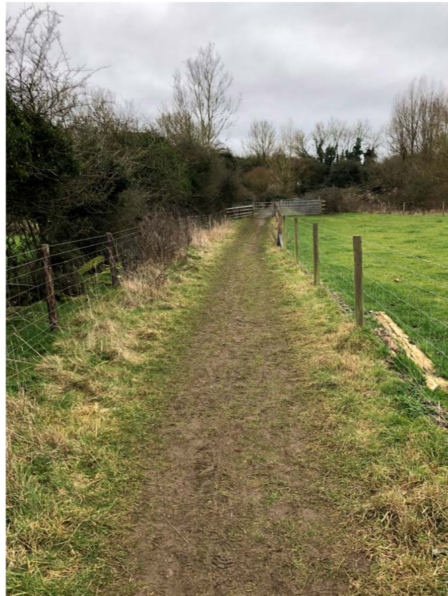
Grassed route requires resurfacing
