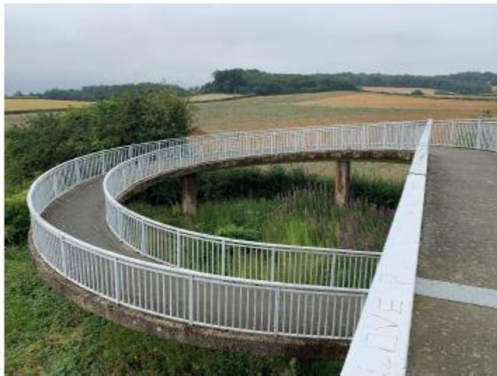
The pedestrian and cycle bridge over Stefen Way is of adequate width for the expected pedestrian and cycle flows and the ramps are of a gentle gradient though the parapets are likely to be below the required height. The bridge is fairly well maintained.
