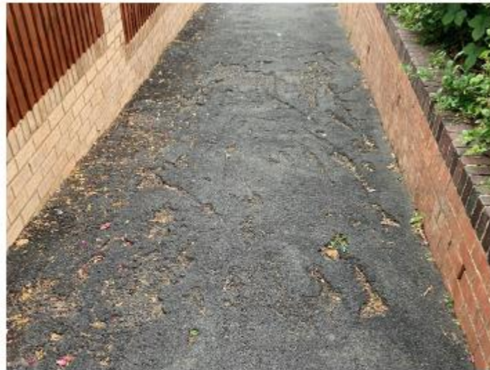
Some paths are in poor condition and require resurfacing.
