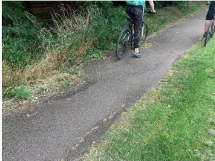
Some sections of the shared facility are narrow and bumpy due to tree roots.
