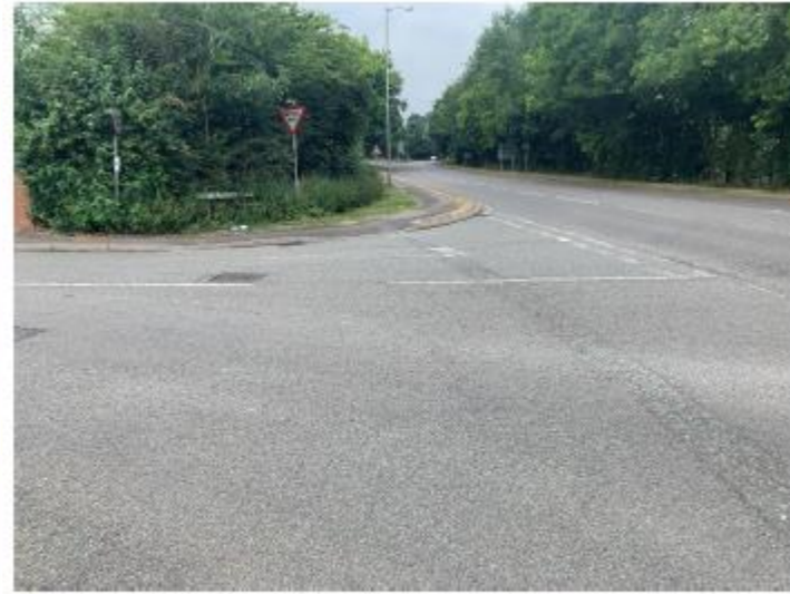
Excessively wide priority junction radii along the route make it hazardous for pedestrians and cyclists.
