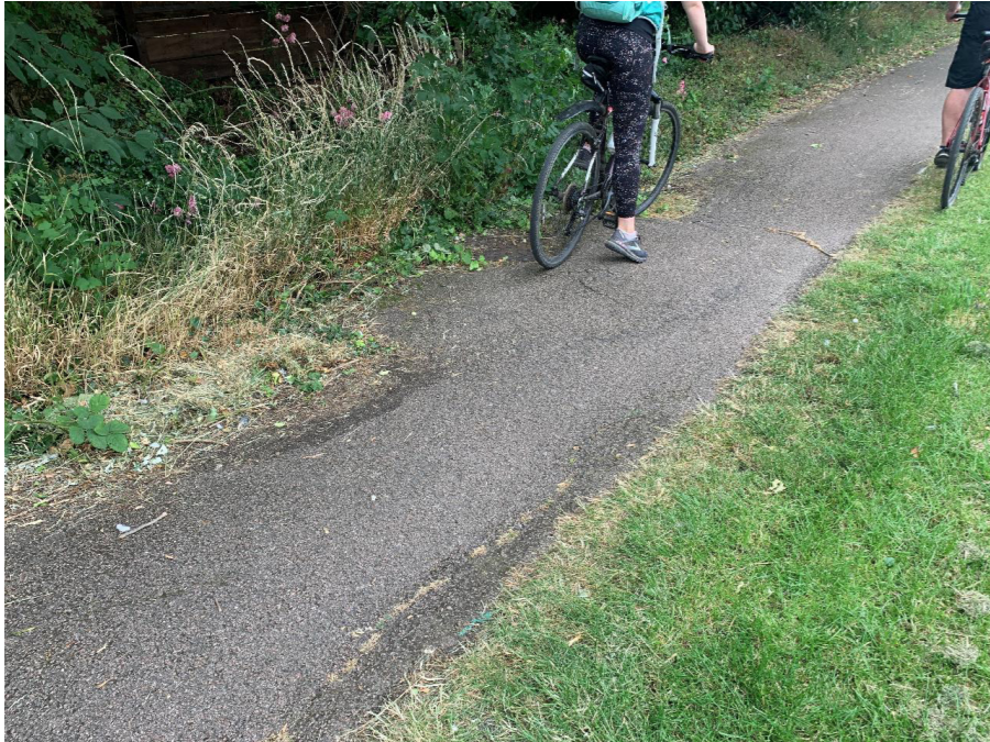
Some sections of the shared facility are narrow and bumpy due to tree roots.
