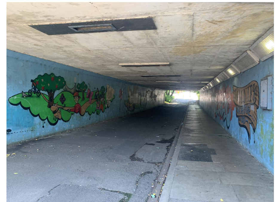
The subway is wide, well-lit, has welcoming artwork and separate space for pedestrians and cyclists, ensuring the subway feels safe to use. A nearby Toucan crossing provides an alternative route to the Icon Innovation Centre (Eastern Way).
