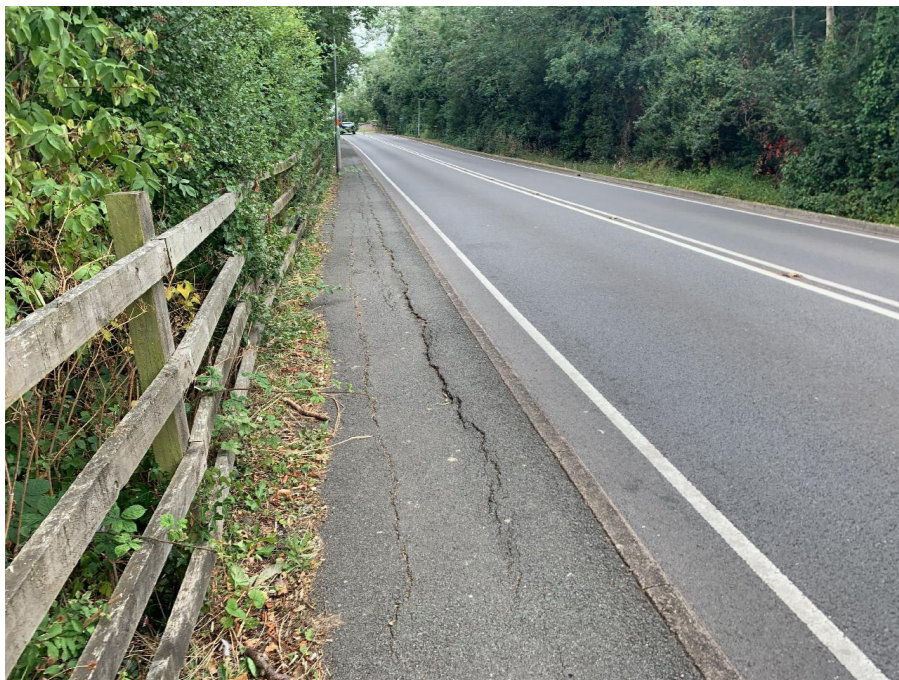
There are some significant defects including cracking in the footway towards the northern end of Ashby Road
