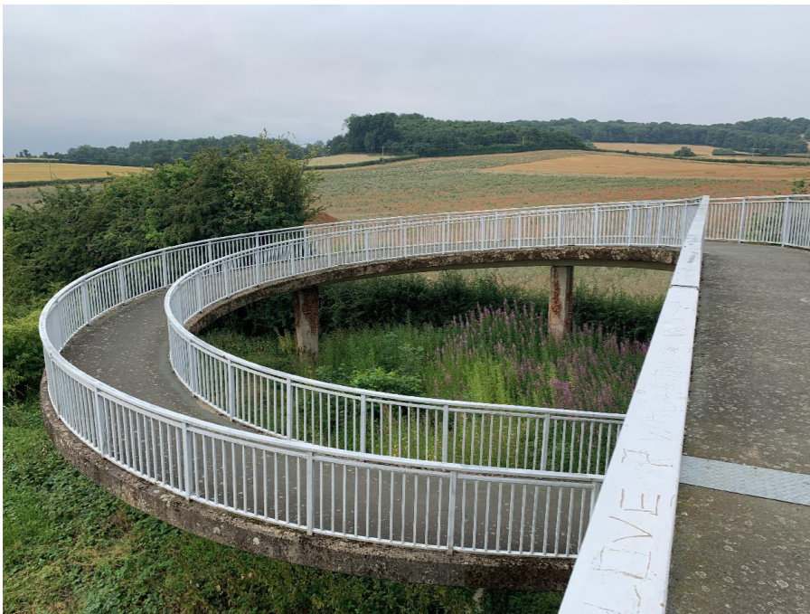
The pedestrian/ cycle bridge over Stefen Way is slightly narrow but provides a gentle gradient which enables cyclists to use it without the need to dismount.
