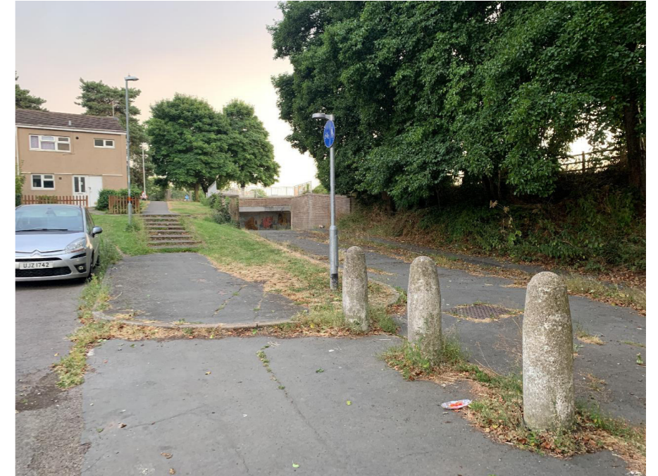
Weeds growing on cycle track surface suggest a lack of maintenance while concrete bollards with no reflectors are a hazard to cyclists at night (Long March/A425 roundabout).
