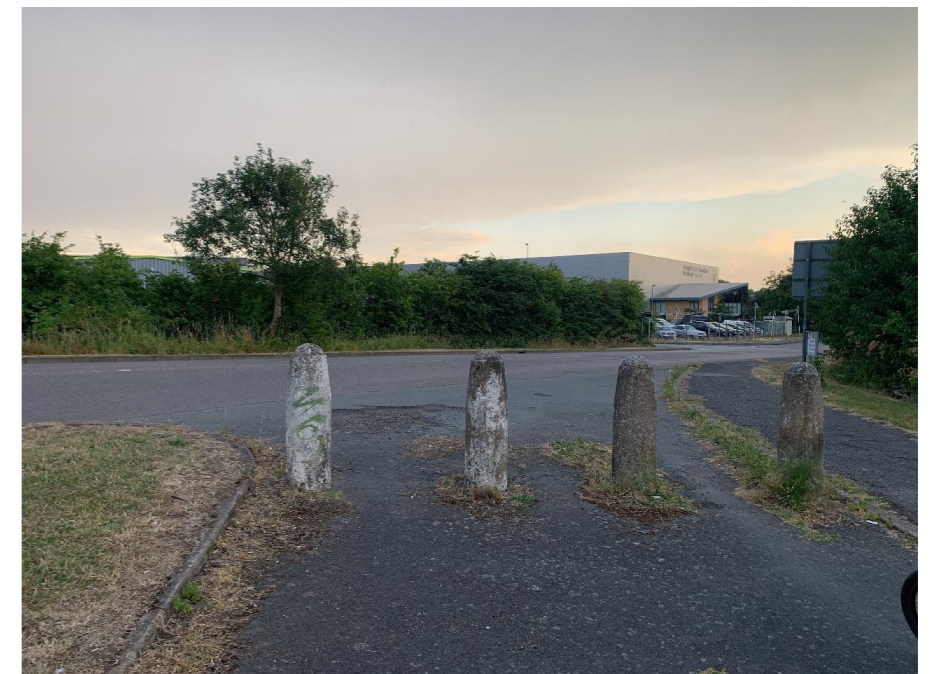
Poor transition between existing facility on the footway and the shared use path under the roundabout via a subway. Inaccessible clearance width between bollards
