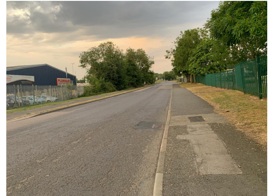
Wide carriageway experiencing higher traffic volumes at peak times. Long, straight geometry facilitates speeding
