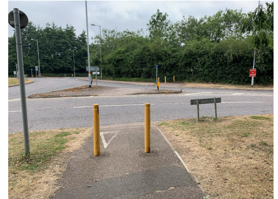
While the ubiquitous slim yellow bollards provide helpful wayfinding, here they are placed too close together on the access and egress to an uncontrolled crossing of a roundabout, creating a hazard for cyclists who are concentrating on traffic.
