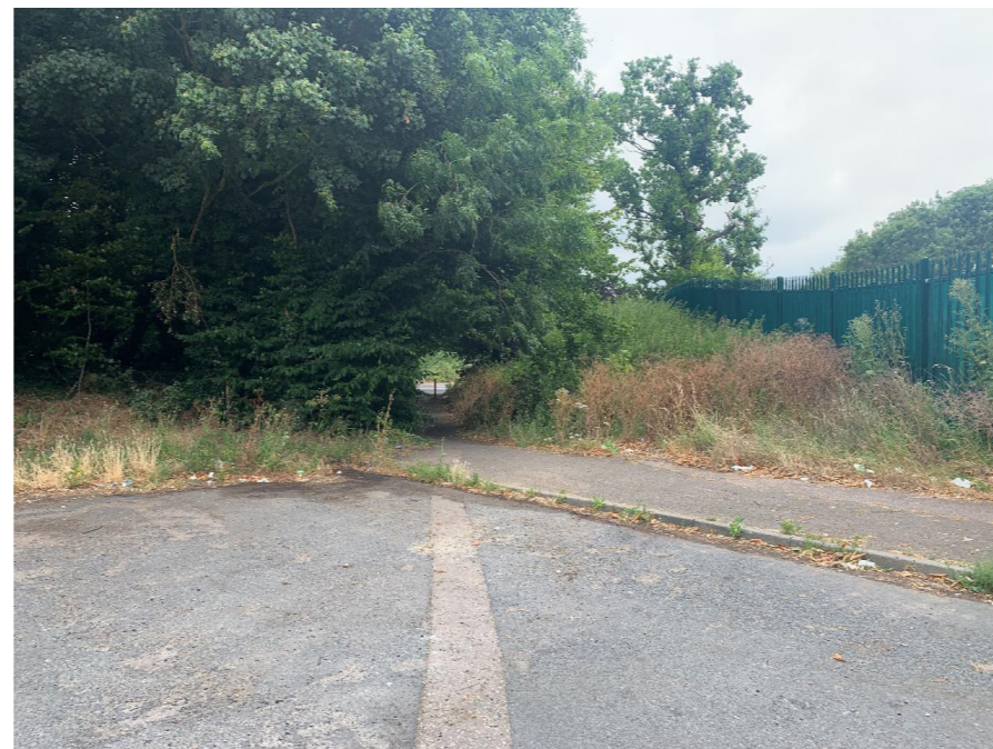
No dropped kerb to access the traffic-free link between Royal Oak Way North and the A45
