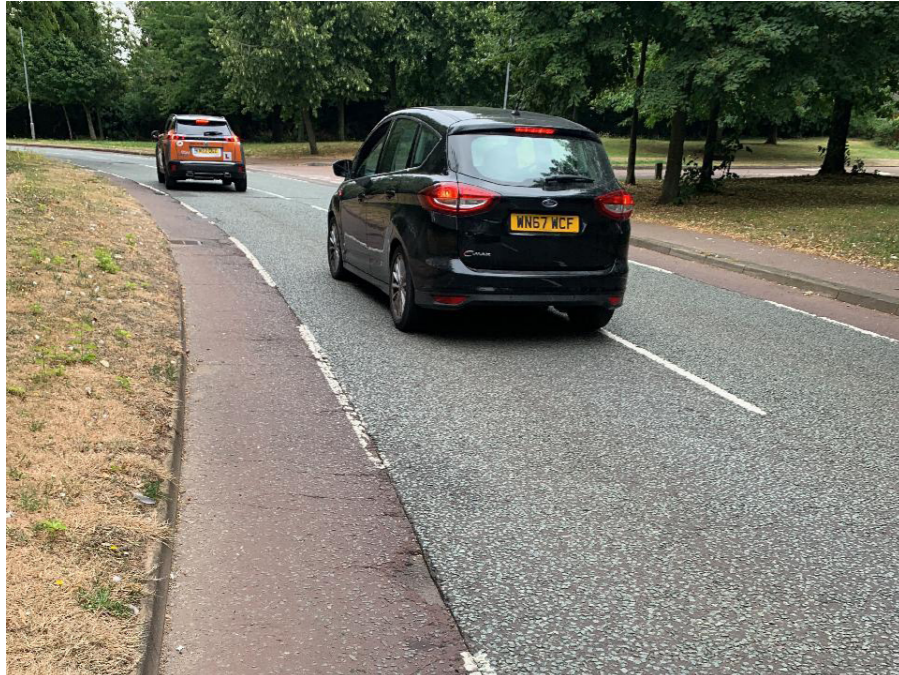
Narrow cycle lanes (in poor condition) and relatively high traffic volumes on Speke Drive create hostile conditions for cycling.
