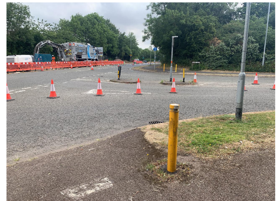
The junction of Ashby Road and Drayton Way is currently a wide priority junction which is hazardous for pedestrians and cyclists.
