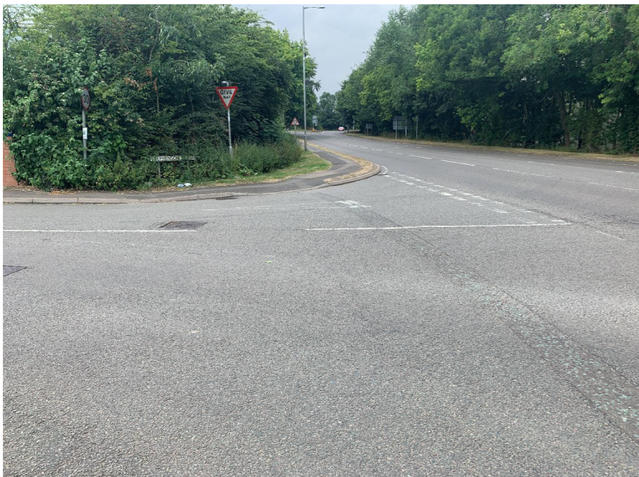
Excessively wide priority junction radii along the route make it hazardous for pedestrians and cyclists.
