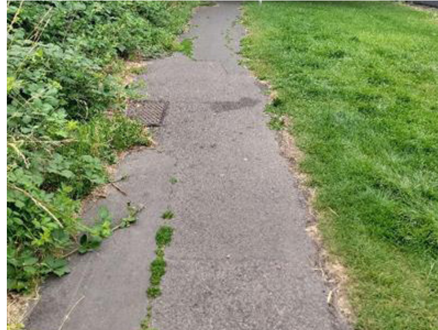
Some traffic-free paths are uneven, creating trip hazards. There is also vegetation encroachment which provides further trip hazards and reduces the effective width
