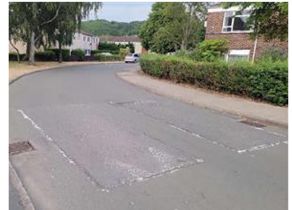
An opportunity missed near Southbrook Junior school to use raised tables instead of speed bumps so that traffic calming measures also provide informal crossing points
