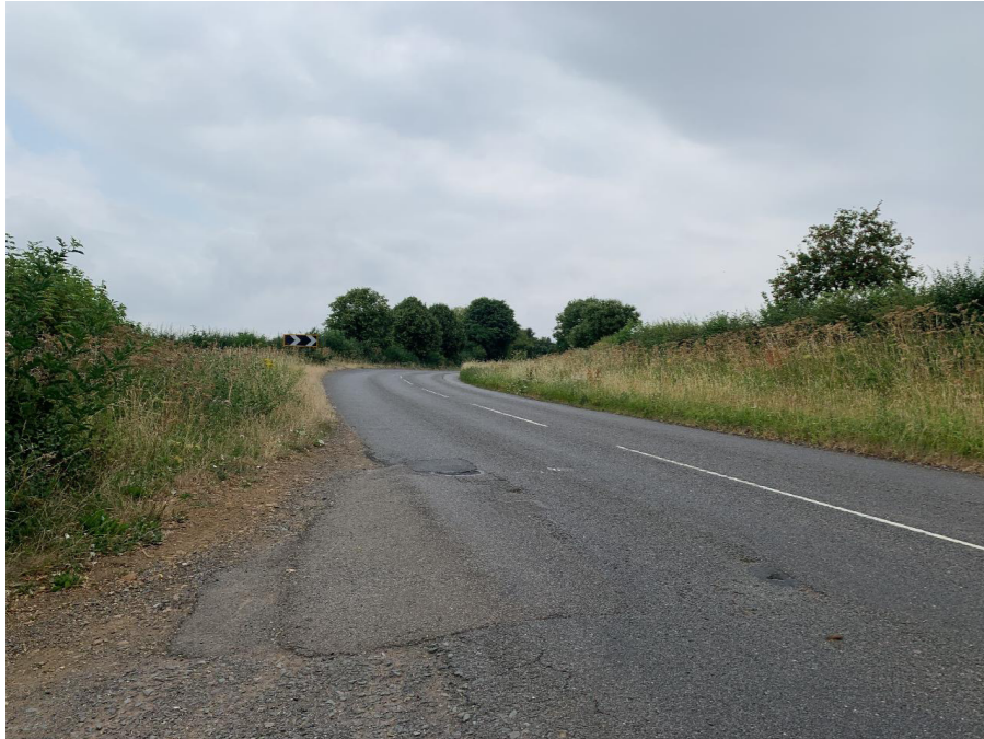
Long Buckby Road is currently National Speed Limit and has no footways or cycling infrastructure.
