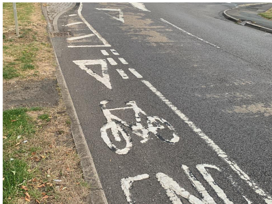
The existing cycle lanes are narrow and end at pinch points such as roundabouts where protection is most needed.
