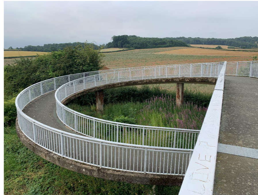
The pedestrian and cycle bridge over Stefen Way is of adequate width for the expected pedestrian and cycle flows and the ramps are of a gentle gradient though the parapets are likely to be below the required height. The bridge is fairly well maintained.
