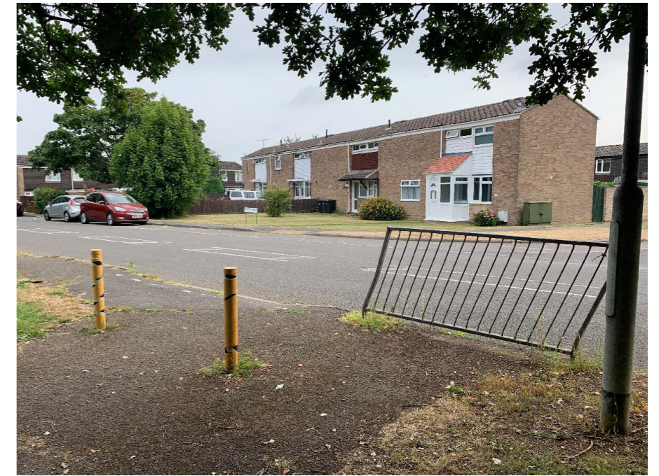
The area at the bottom of the ramp is untidy and has the potential to bring pedestrians and cyclists into conflict. The uncontrolled pedestrian crossing is in poor condition and lacks tactile paving on the south side.
