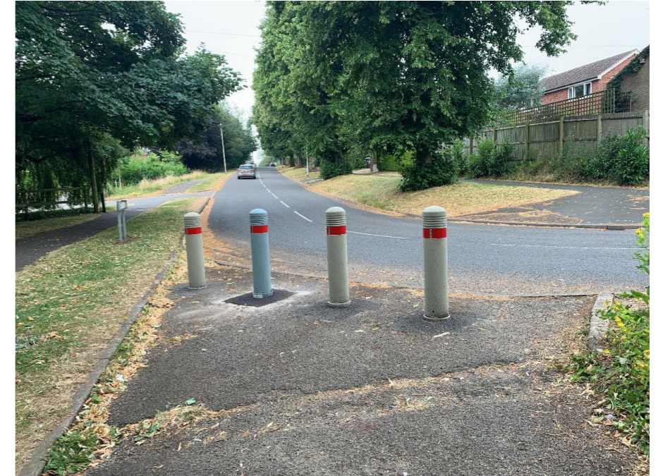
The entrance to the ramp on the southwest side of the subway is on a bend with the bollards placed too close together and the surface in poor condition which could lead to collisions or falls.
