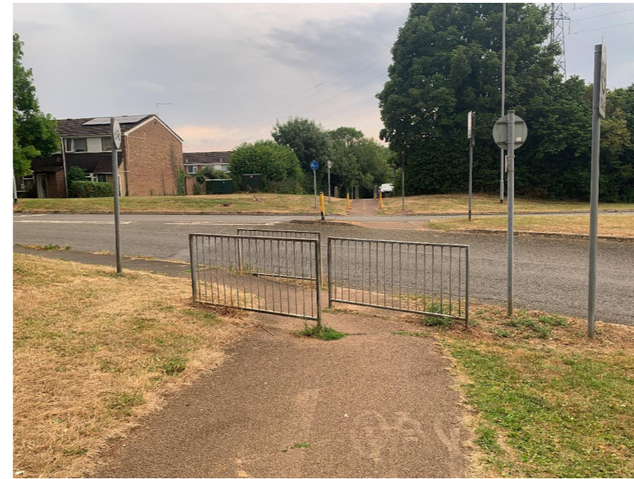
Barriers on the cycle track adjacent to Eastern Way make it difficult for people cycling or using wheelchairs or mobility scooters to access the dropped kerb.
