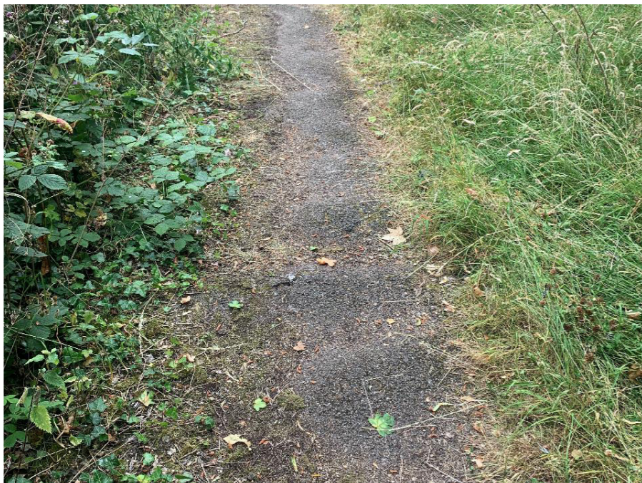
At the junction with Daventry Road, the path diverges from the road, emerging on Daventry Road well away from the junction which helps support a safe transition to the carriageway. However, the path is narrow, bumpy and overgrown.
