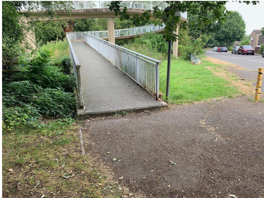
There is a large lip at the bottom of the ramp which will make it inaccessible for wheel chair and mobility scooter users as well as some cyclists, particular disabled cyclists and people using non-standard cycles which tend to be heavier.
