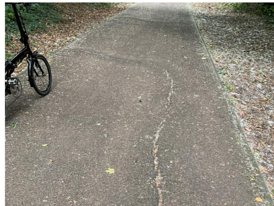
There are some short sections along the disused railway line where the surface has cracked and others where tree roots have damaged the surface and made it uneven which could cause a trip hazard for pedestrians and make the route uncomfortable for cycling and scooting, particularly for disabled cyclists.
